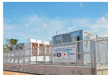
First energy-efficient data center in Laos
